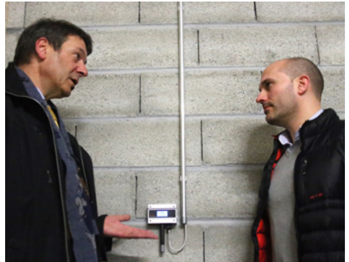
Marc Golay from Ports France Genève shows Marcel Rohrbach from Rotronic where one of the Rotronic transmitters is mounted.
