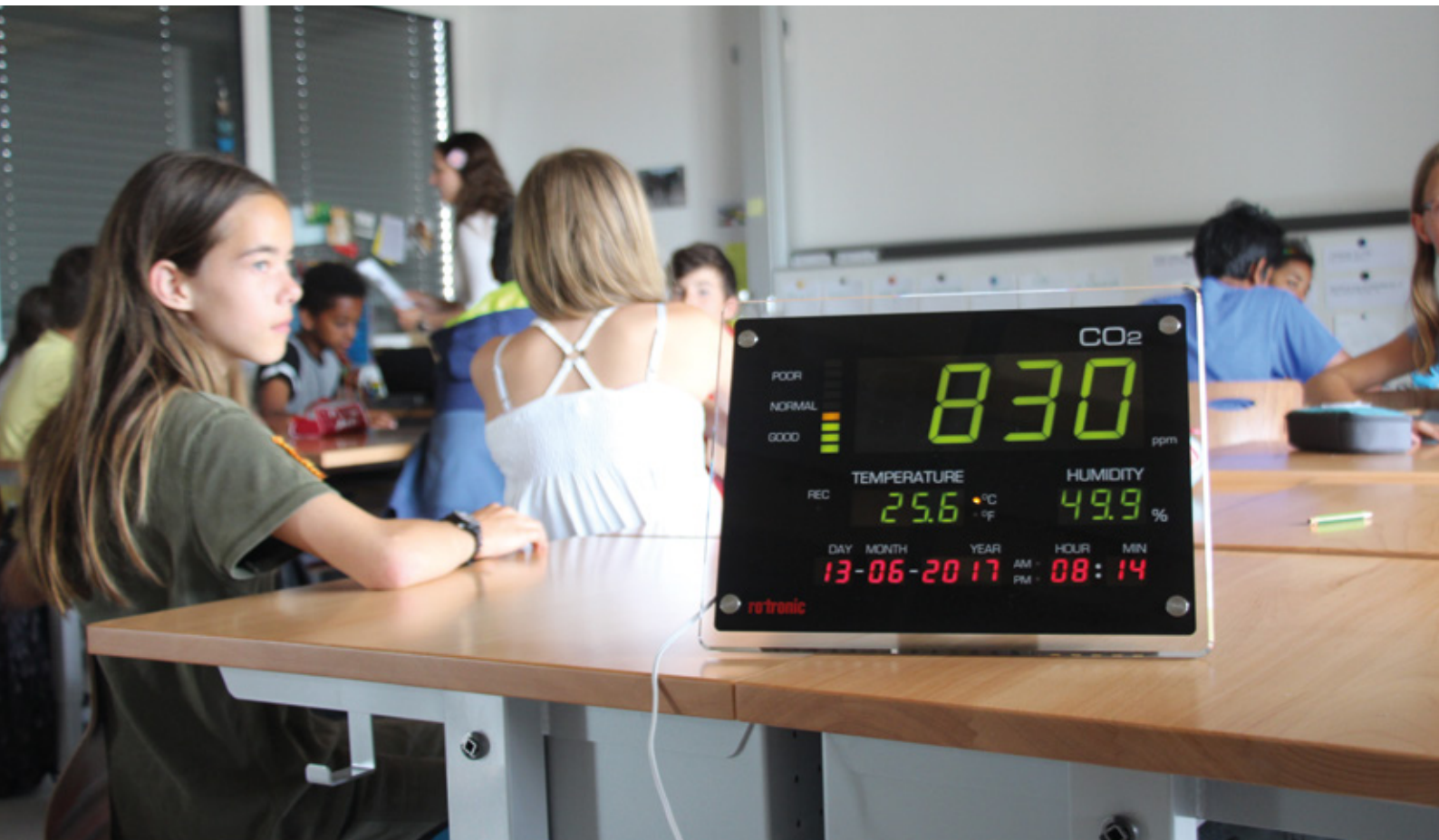
CO 2 display from Rotronic in use in Class 5 / 6B at Köniz-Buchsee Primary School (Switzerland).
