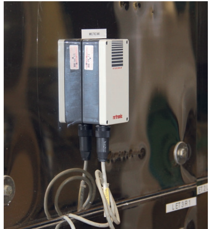
Rotronic I200 sensor, providing reliable service for more than 15 years.
