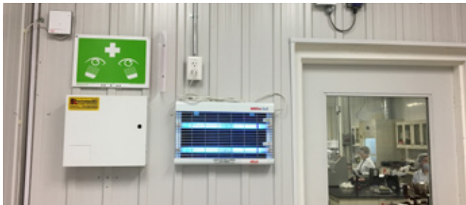
Differential Pressure Monitoring of the Labs.
